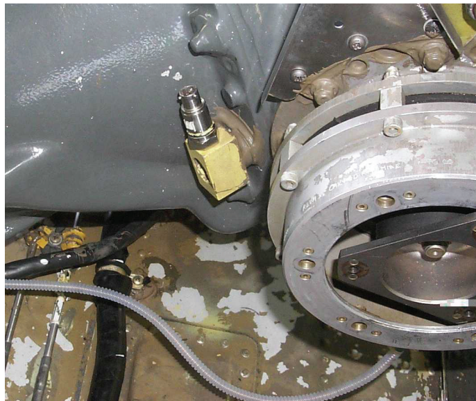
Figure 19. No. 2 Input Module Accelerometer Installation (ACC2)
