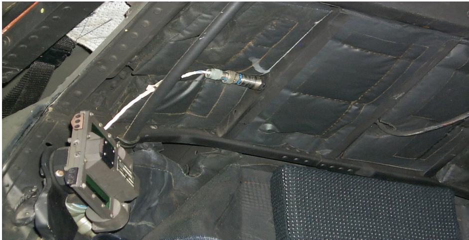
Figure 3. Lateral Accelerometer Installation (SPU/External Wiring)
